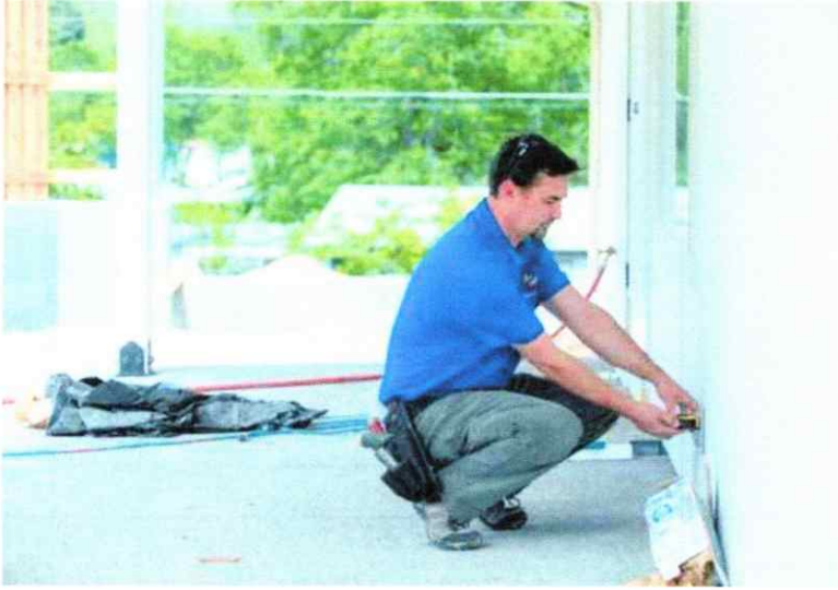
Halvorson checks an electrical outlet outside a new home still under construction.
