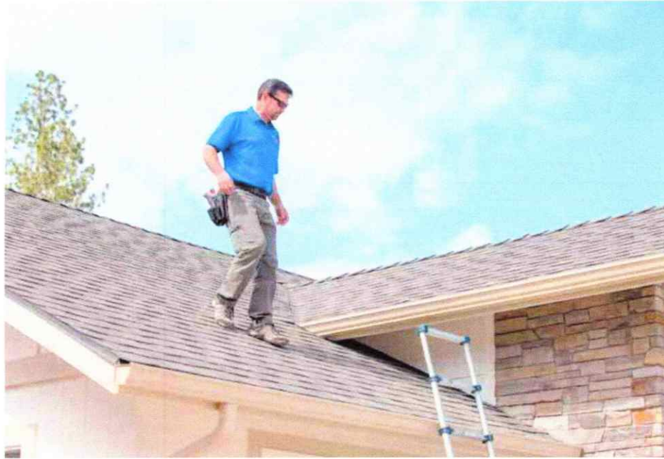
Thorin Halvorson, home inspector and owner of Southern Oregon Home Inspections, checks out the roof of a new home still under construction on May 1 in northwest Grants Pass. He suggests an inspection before homeowners put their place on the market.
